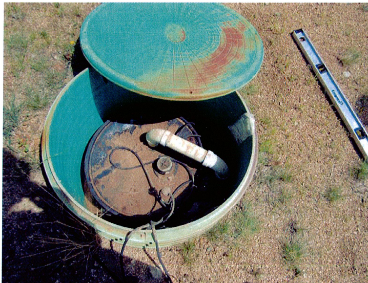
Grinder Pump at South East Corner
