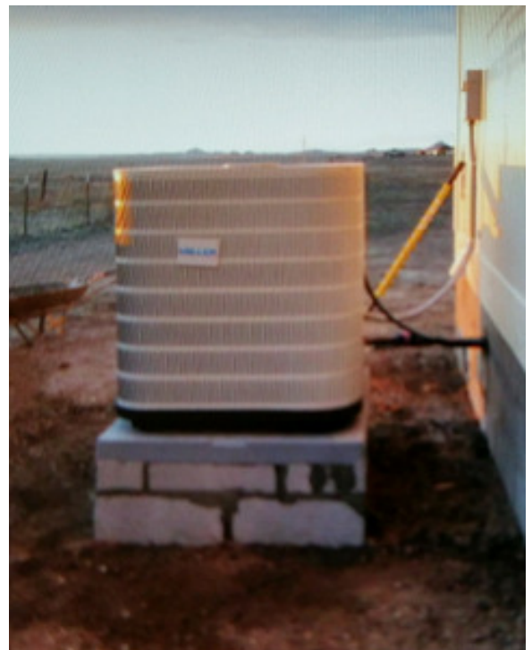
Raised A/C Unit, Date Taken: 5/3/2016
