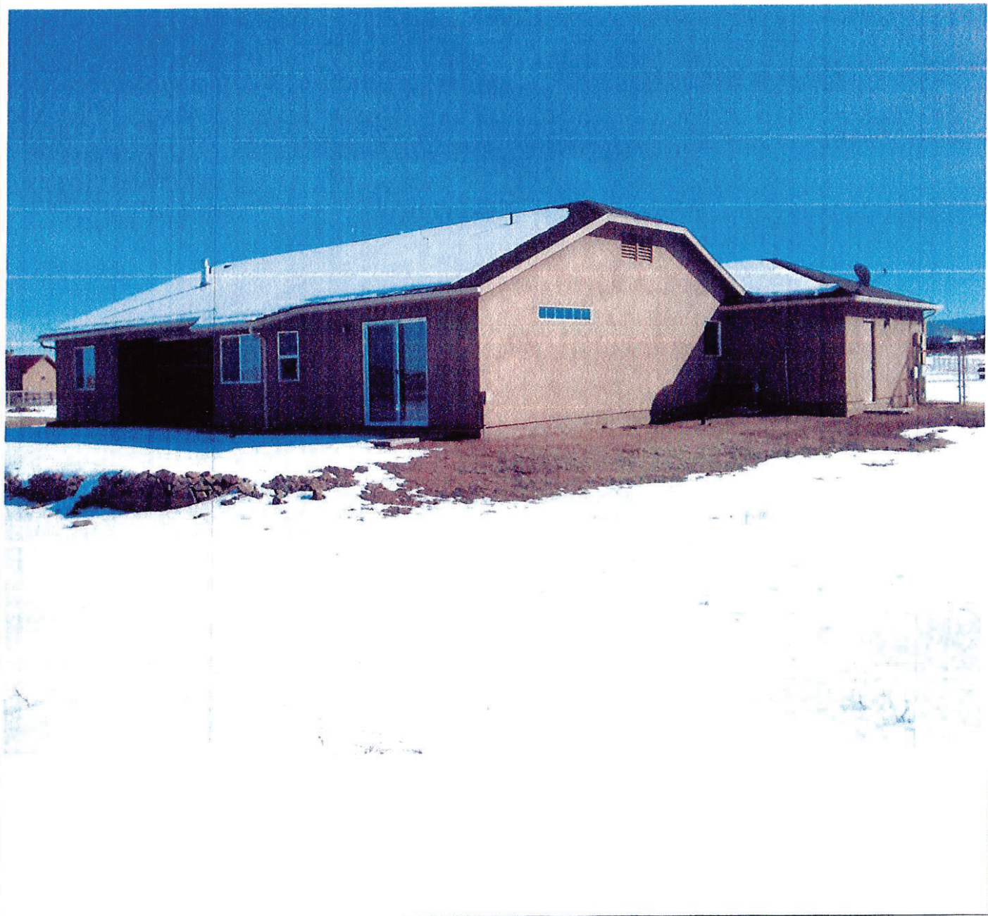
SOUTHWEST END & NORTHWEST SIDE – C2E A/C PAD IN BLDG. NOTCH BELOW SINGLE WINDOW AT REAR OF ATTACHED GARAGE
