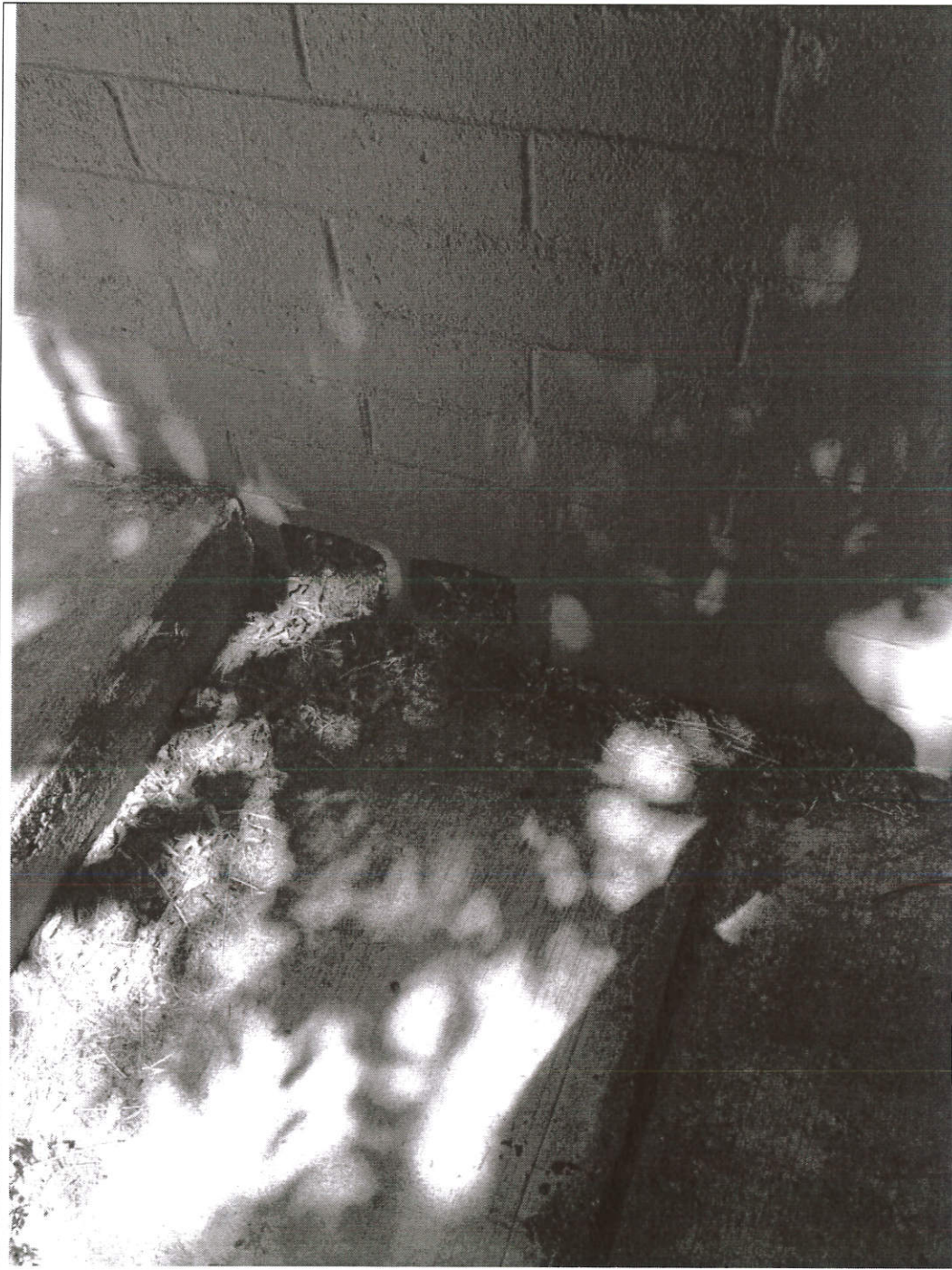
Flood opening on East side
