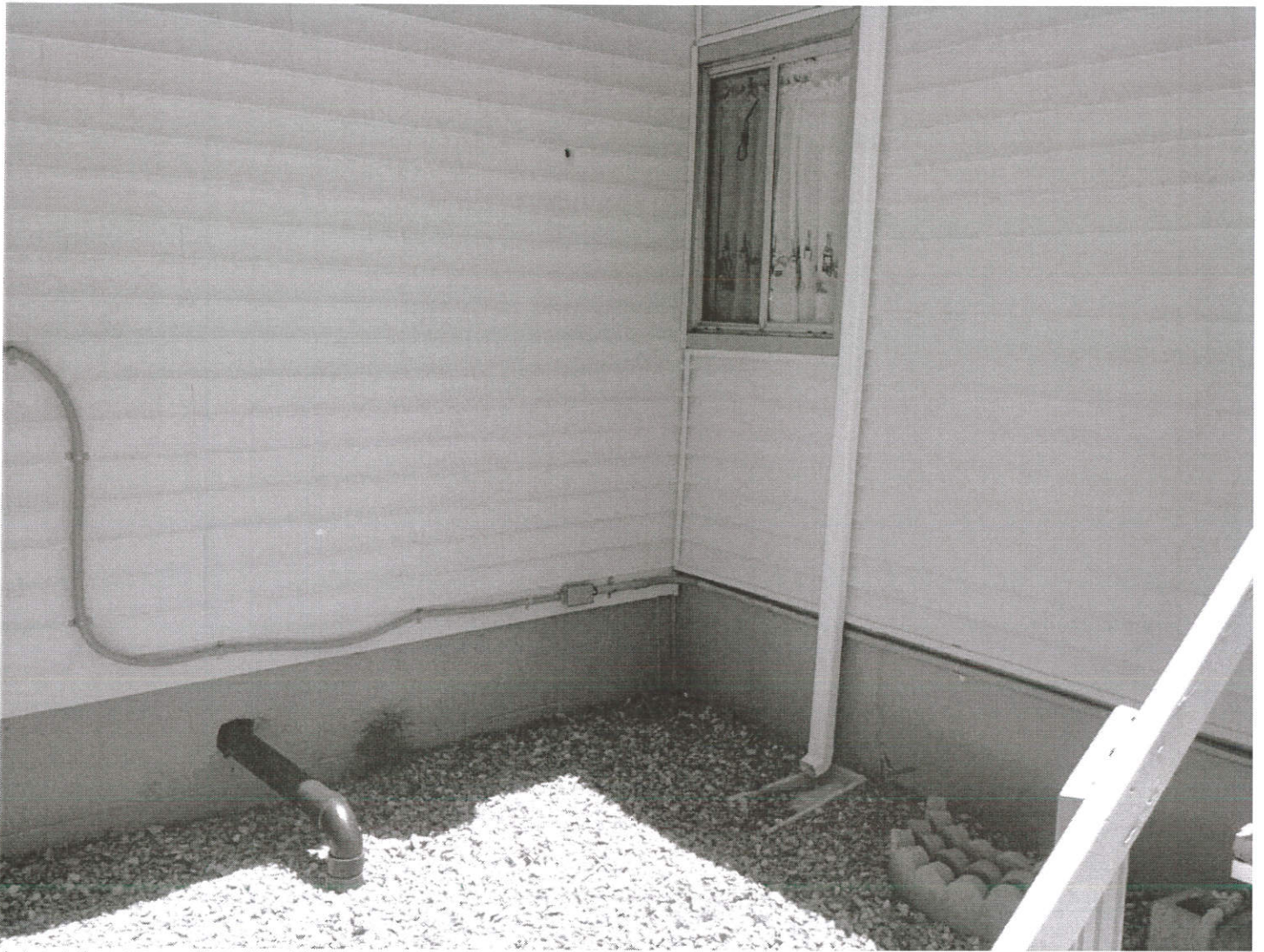
Joint at the stem wall and mobile home skirting on the North side of the house
