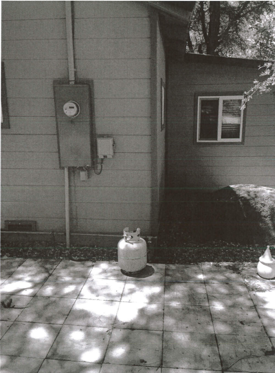
East side of house, Right side, 05/29/15 (Next higher floor, electric panel, flood vent)
