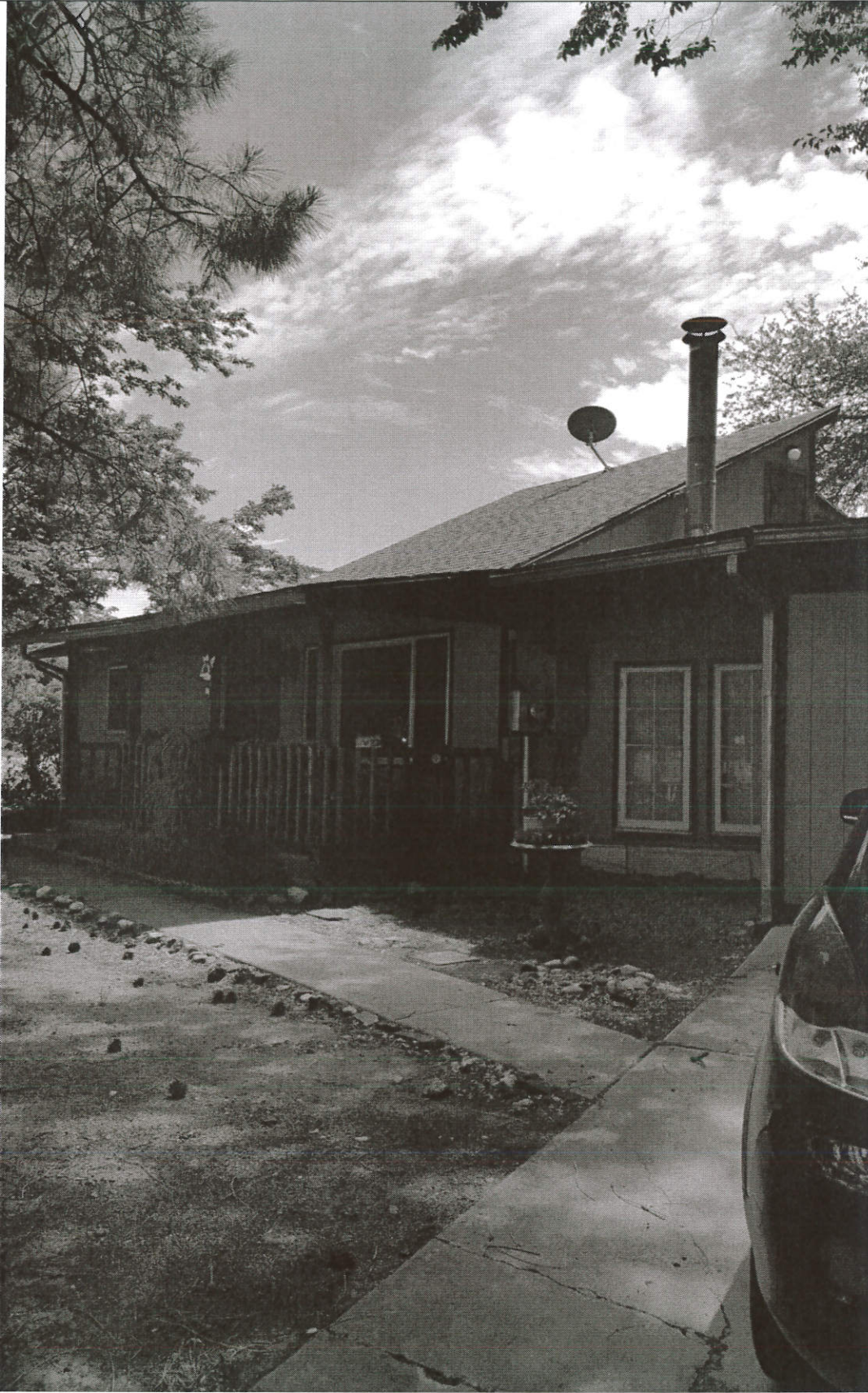
Electric panel on the main house
