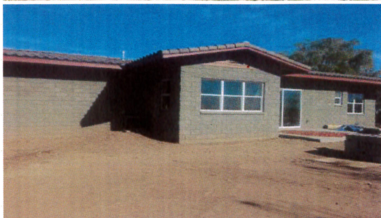
AC UNIT BACK OF HOUSE 11-20-15
