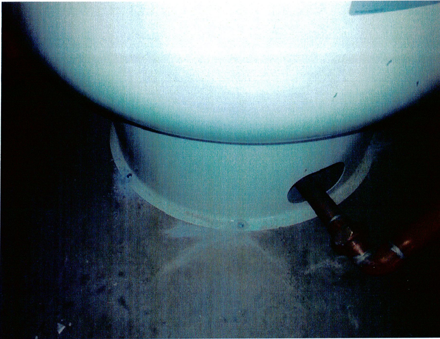
WATER PRESSURE TANK ANCHORED
