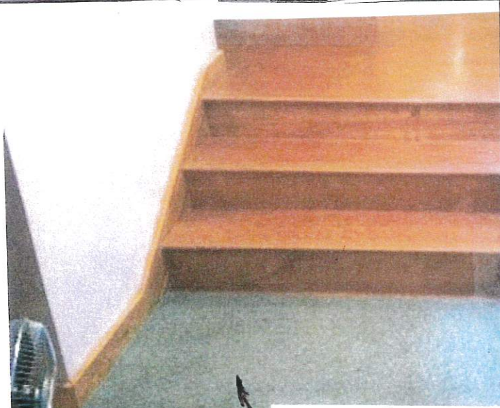
PHOTO #2, LOOKING WEST AT JOINING OF ORIGINAL HOUSE TO INSIDE STEPS TO FIRST FLOOR OF ADDITION
