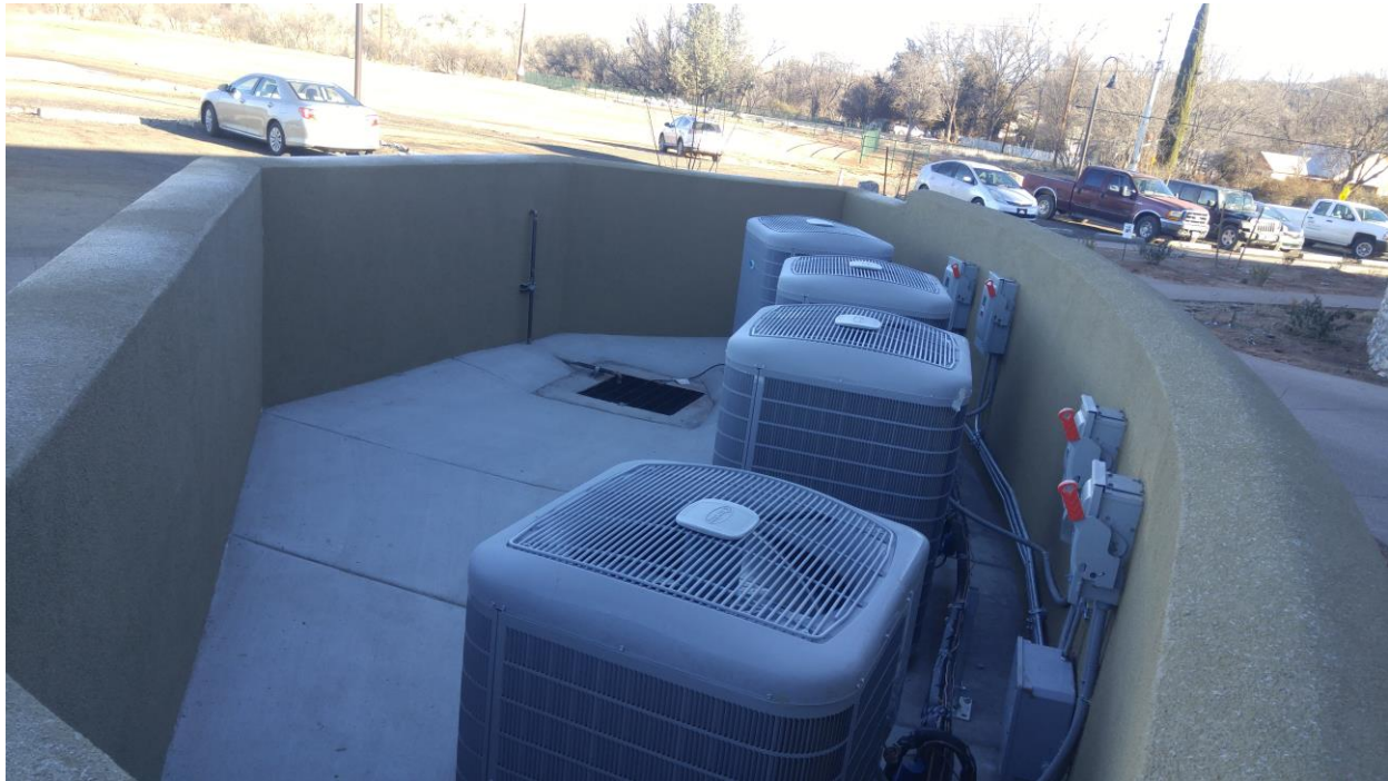
HVAC – Left Side
