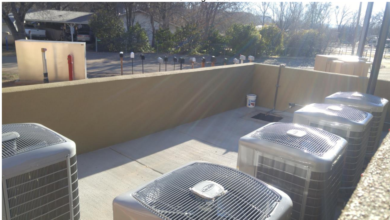
HVAC – Right Side
