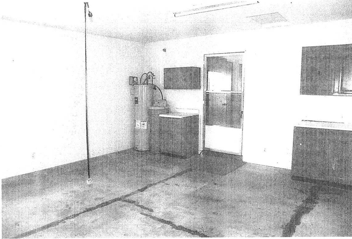
WATER HEATER & SOFTENER IN GARAGE
