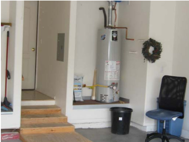
--ELEVATED H/W HEATER GARAGE
