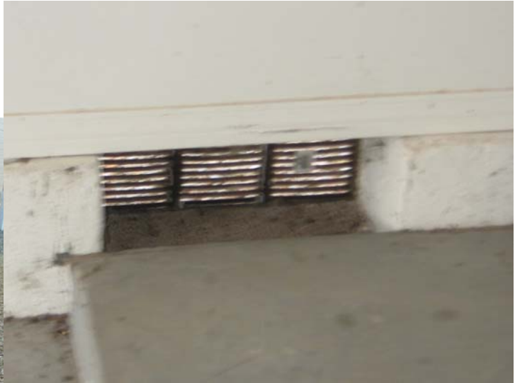
--GARAGE FLOOD VENT
