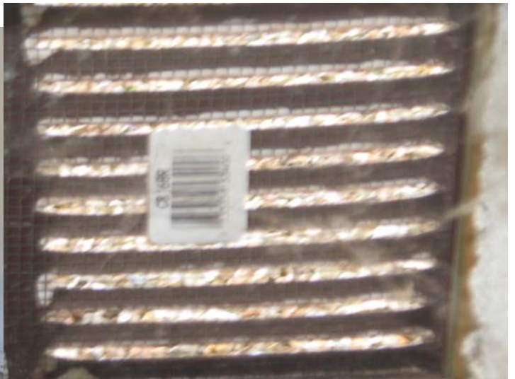
-- CLOSE UP BAR CODE ON VENT COVER
